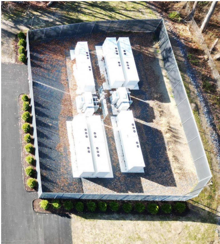
Figure 2: Calibrant Energy 4.9MW BESS Project, Westchester, NY
