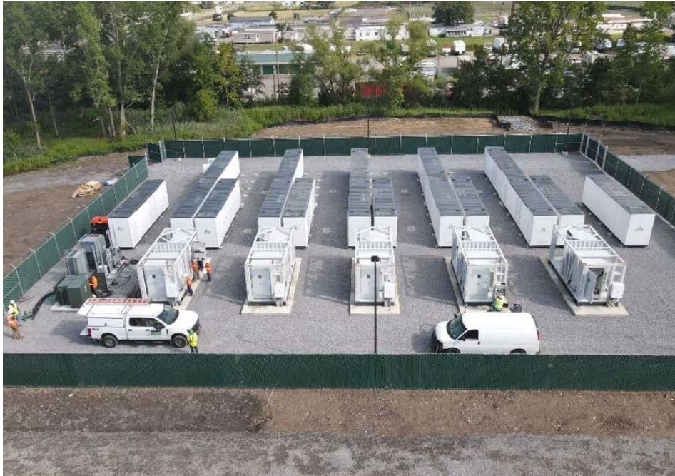
Figure 1: Key Capture 20MW BESS Project, Blasdell, NY
